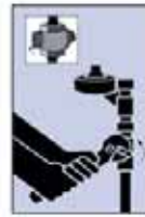
Close-up of a typical gas valve
